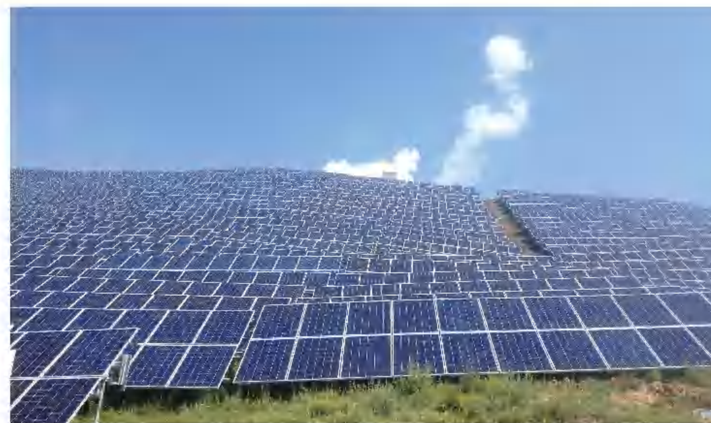
Hebei Baoding Mountainous Solar Power Plant Project
