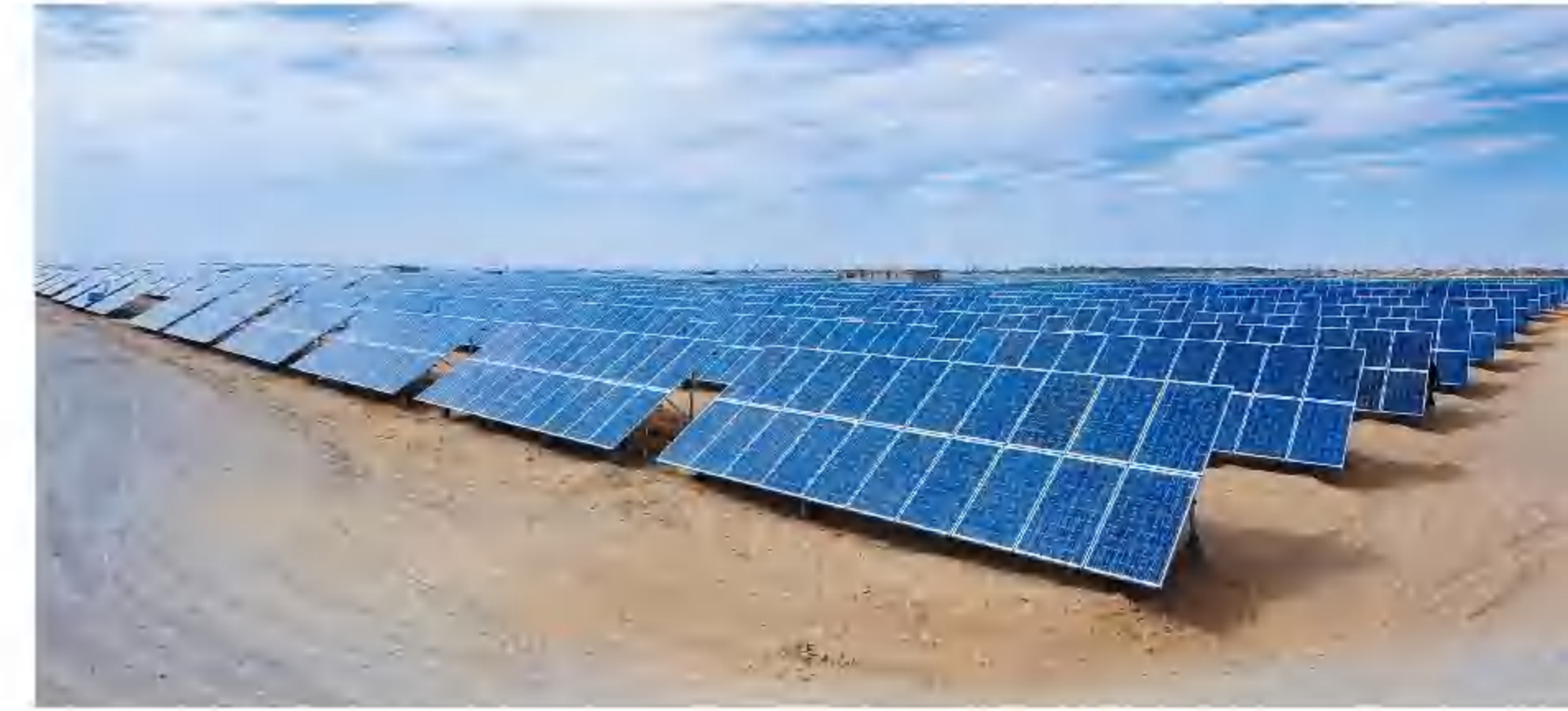
Qinghai Golmud Solar Power Plant Project
